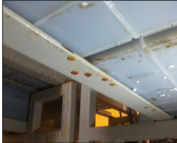
Figure 4: Droplets of Electrolyte can be seen below the cell seats, the seats are basic L-sections made up of steel coated with enamel or epoxy paint.
