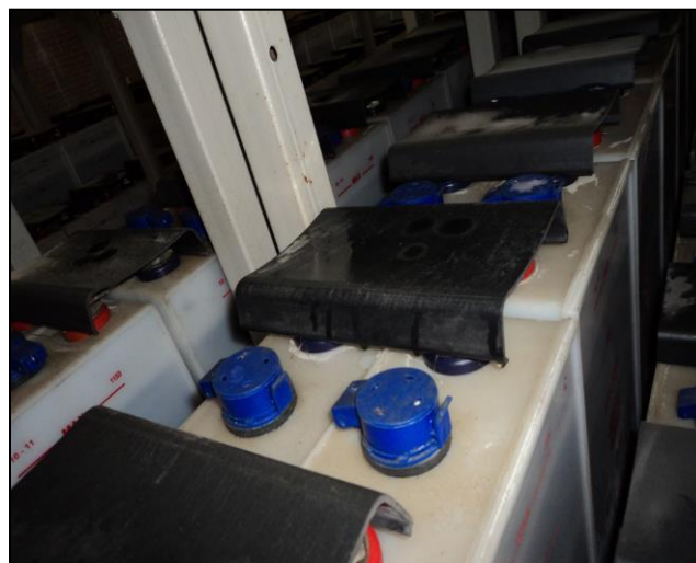
Figure 5: Electrolyte can be seen on top of the covers of the terminal links.
