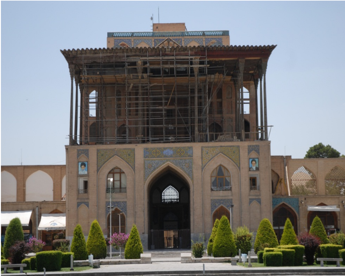
Figure 2. Ali-Ghapoo Palace from outside view; the restoration of the monument is seen in this figure.
