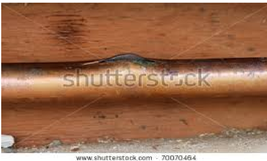
Figure 1:Showing a crack in the oil-pipeline. Source Shutterstock.com
