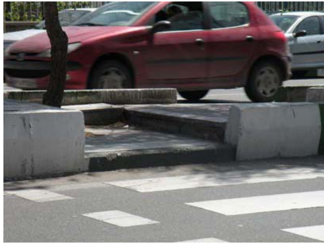
Fig.2. level is inconsistent between the two street sides at a pedestrian crossing place
