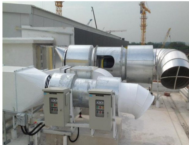
Figure 2: Outlet Exhaust Fan in Industry [7]
